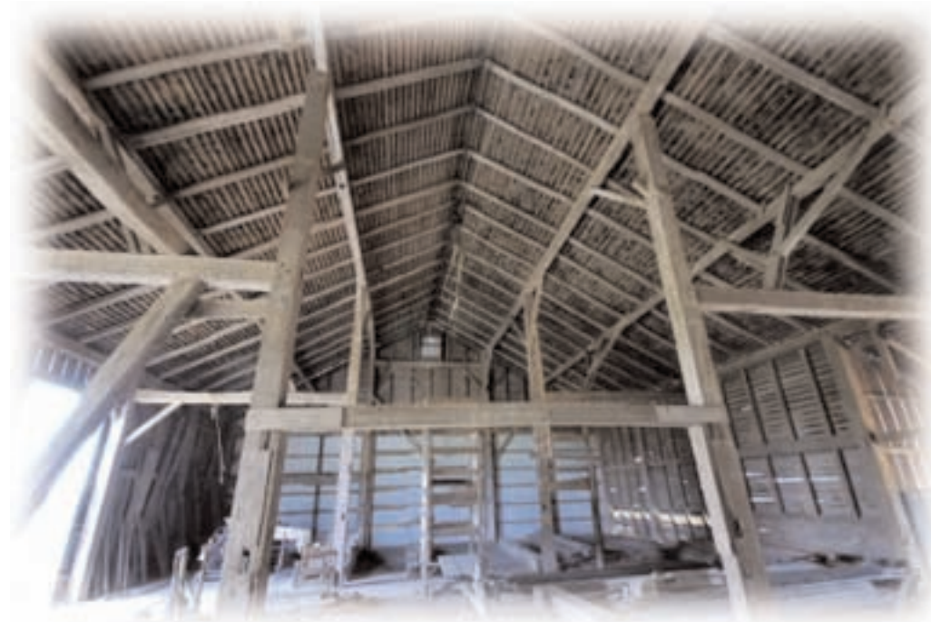
Bracing and roof structure of one of the barns on the tour during Ohio Barn Conference X. For more information, please see the foldout centerfold in this issue.
