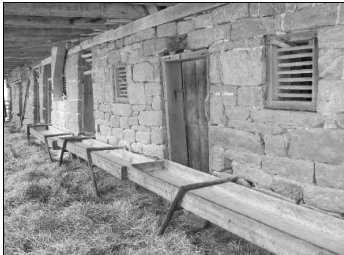
The Poorman barn in Perry County exhibited some outstanding features. This stone wall provides entry to the horse stables beneath the forebay of the barn. Below: The Poorman barn on SR 13 in Perry County is a double framed Pennsylvania bank barn with some of the logs cut in 1818 and 1819. Inset: This nameplate hangs on the gable end of the Poorman barn.
