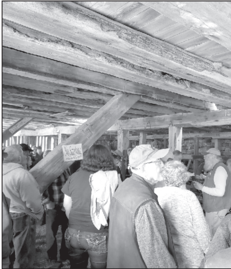
Rudy Christian (at far right) in the Pershing Barn basement discussing the giant timbers that make up the floor system.
