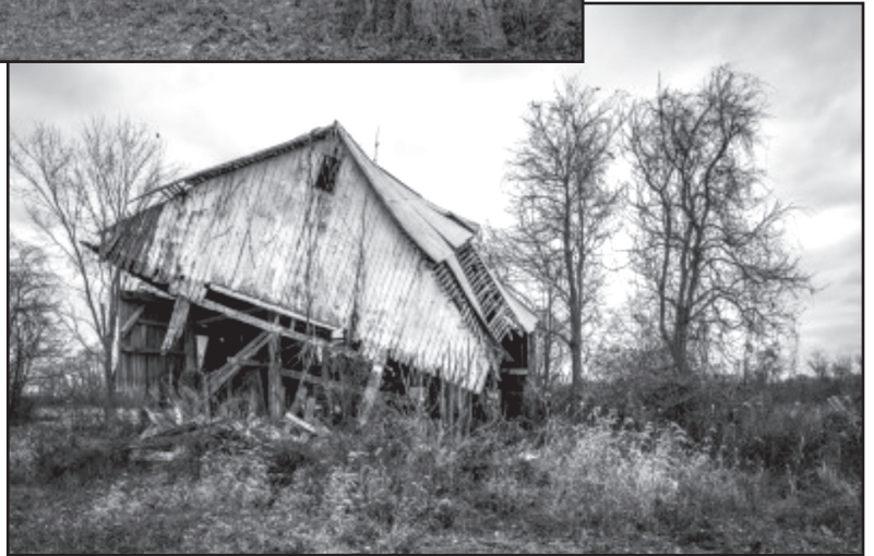
The old barn leaning heavily to the southwest.
