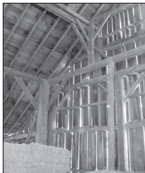
Interior view of barn that shows some very rare ‘doubling up’ of timbers.
